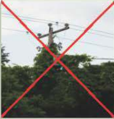
OVERGROWN VINES AROUND ELECTRICAL EQUIPMENT
